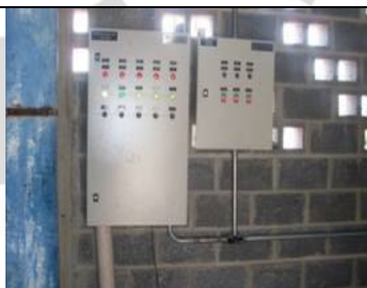
Painel de controle ETE
